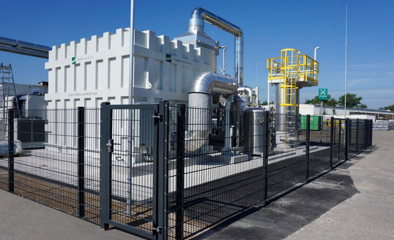
Fuel cell power plant on the FRIATEC site.
