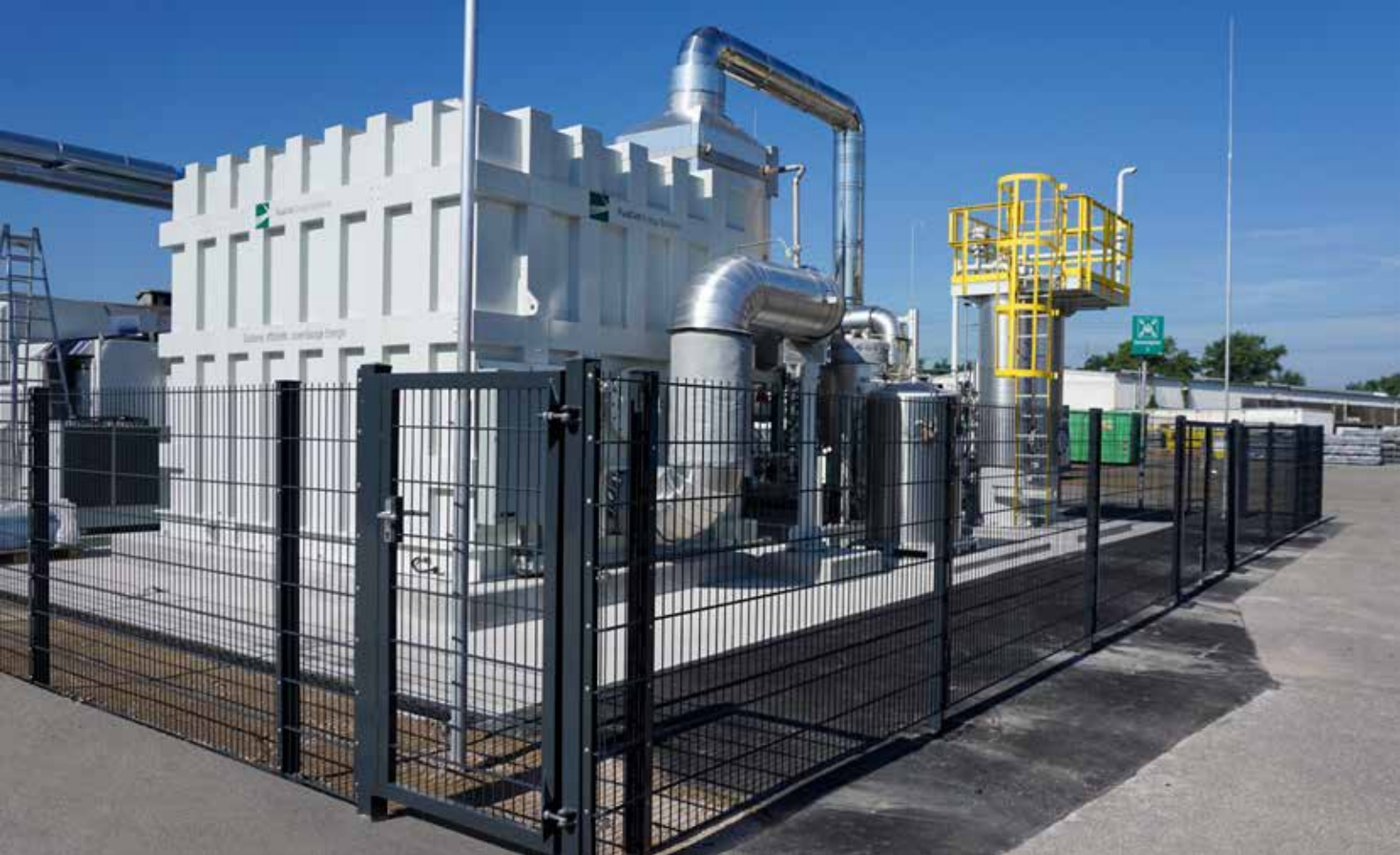
Fuel cell power plant on the KYOCERA Fin ceramics Solutions GmbH site.
